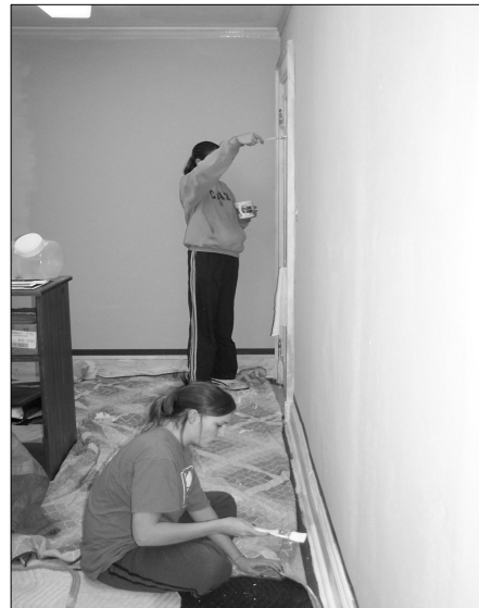
Maggi and Jessi working in the Youth Room. Stop upstairs & see the progress that has been made.
